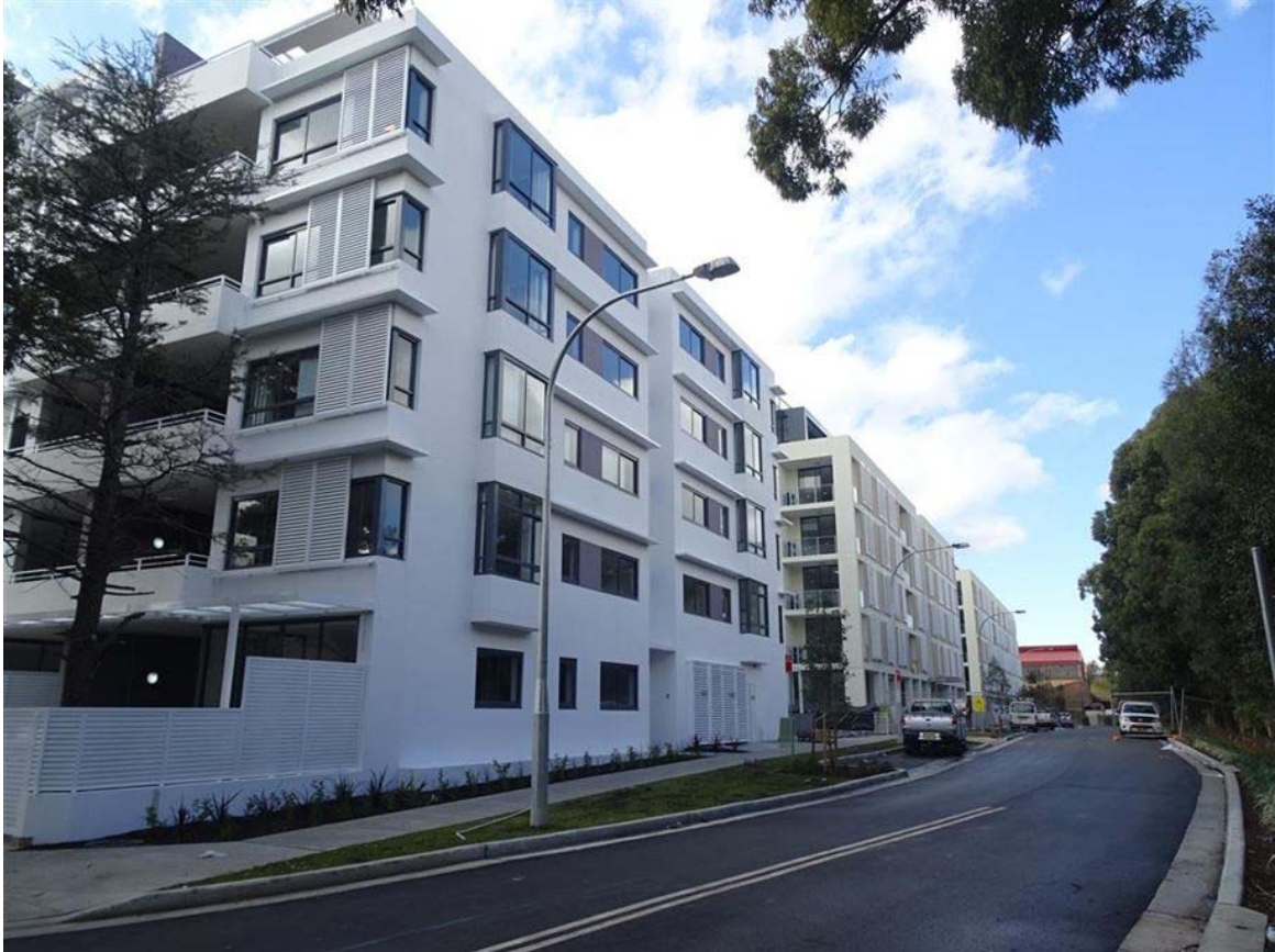
Figure 8: The southern edge of the site showing Buildings D, G and H nearing completion.
