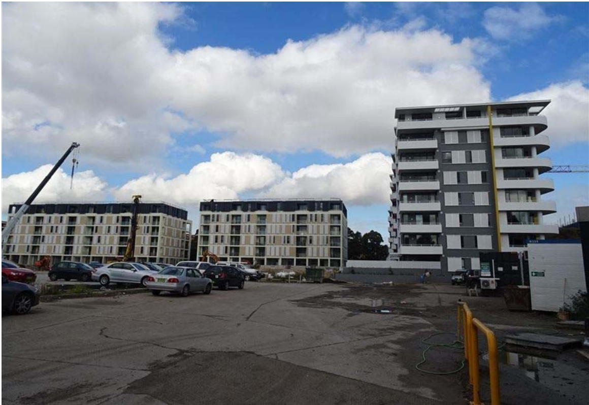
Figure 6: Looking south across the site showing Buildings H, G and D nearing completion.
